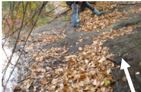
Sediment deposition and walkway washout along the banks of the Muddy River; the original river bank is shown by the arrow.
