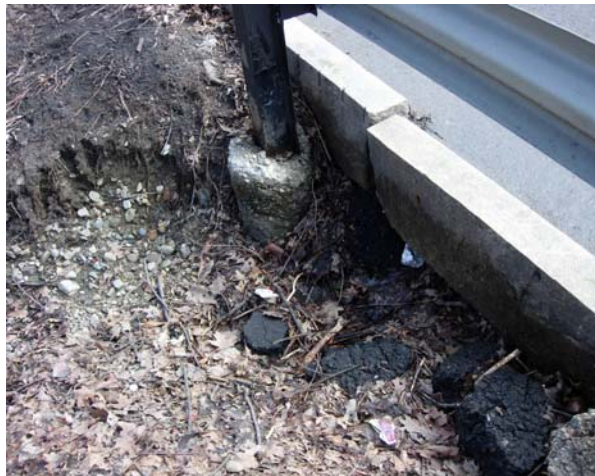
Figure 3: Riverway curb compromised across from Wheelock College, 3/28/07
