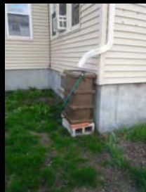
Rain Barrel in use along Nichols St. - Everett
