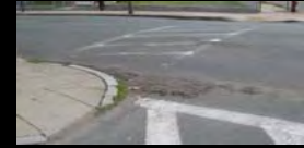
Sediment accumulation Washington Ave. - Chelsea
