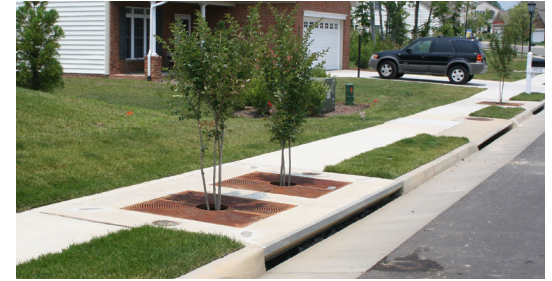
Tree pits consist of an underground structure which collects and treats stormwater.
