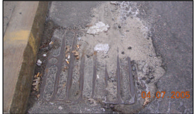
After years and years of neglect, the debris in this DCR stormdrain has entirely filled the catch basin, rendering the drain completely useless.
