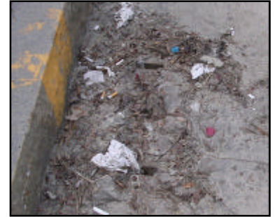
This catch basin, on the ramp leading to Storrow Drive, Westbound, is so clogged that you can barely tell there is a stormdrain beneath the debris.
