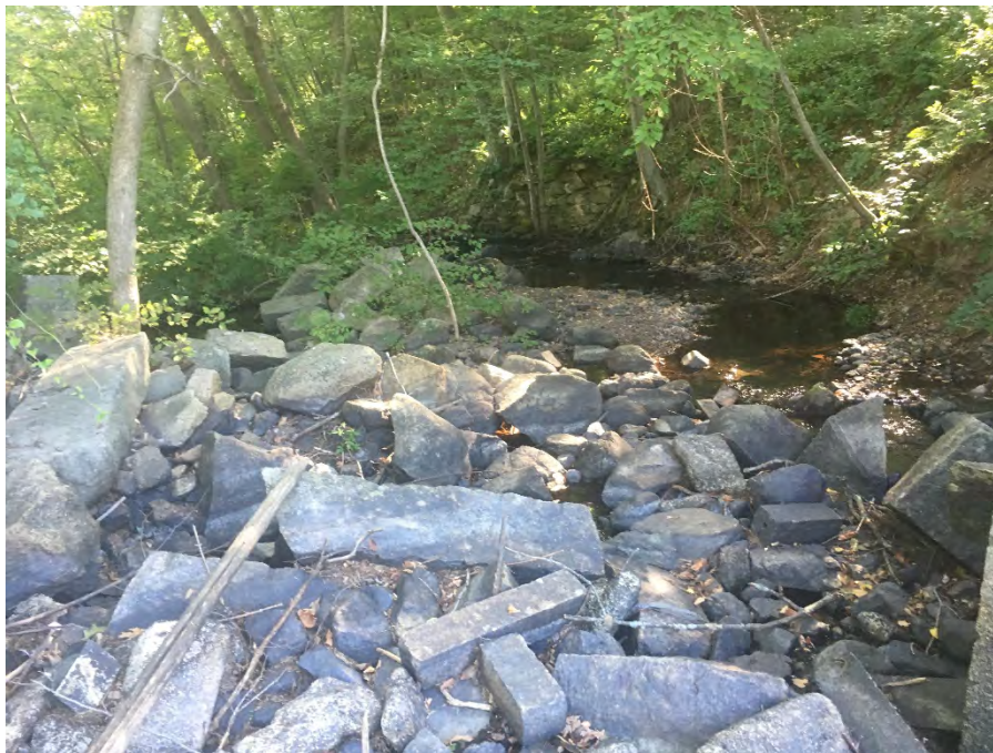
Photograph No.: 4 Rubble and debris within channel below spillway-Eagle Dam
