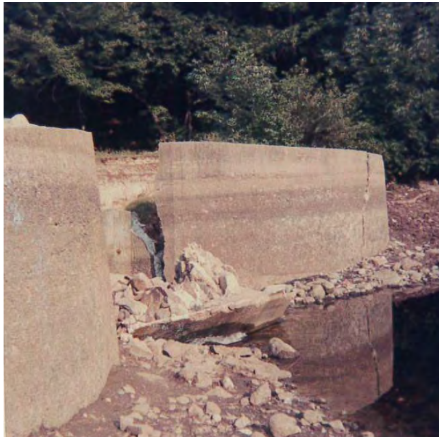
Figure 3. Eagle Dam Failure c.a. 1972 (source Town of Wrentham)
