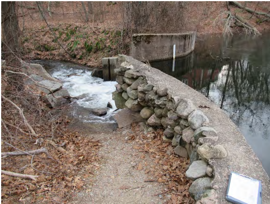
Photograph No.: 2 Erosion behind western retaining wall-Eagle Dam
