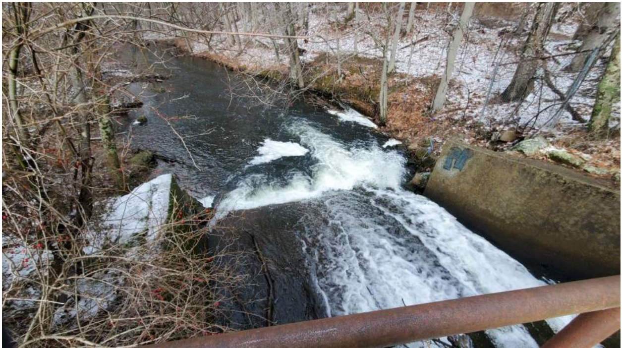
Photo 8: Bush Pond Dam (MA01158) looking downstream at the discharge channel from the pedestrian bridge above the spillways.
