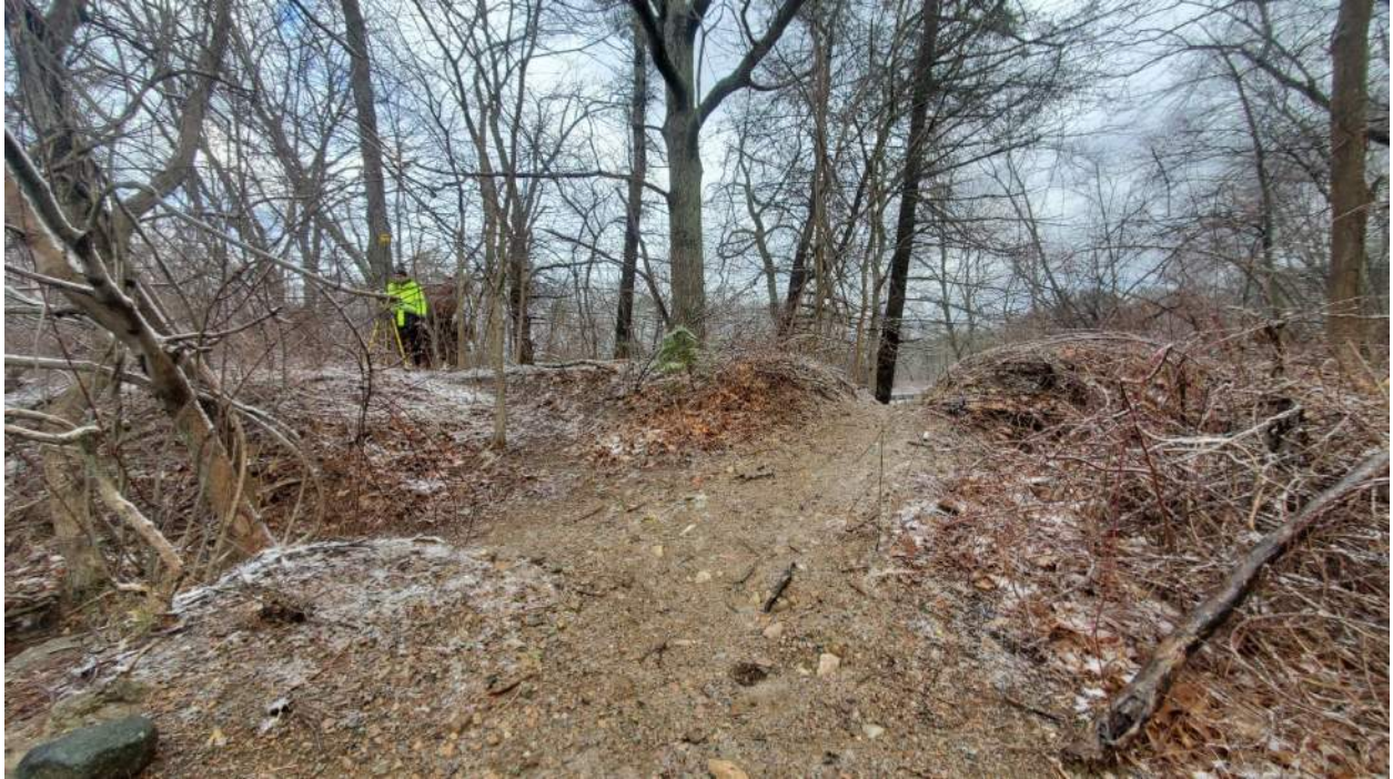
Photo 1: Eagle Lake Dam (MA02263) Embankment looking downstream. Eagle Lake Dam's embankment ungulates with several eroded walking paths, as seen in this photo.
