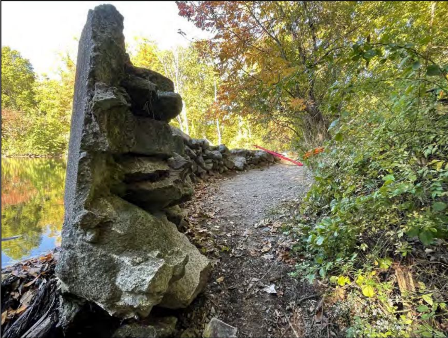
Photo No. 9.: Erosion of the dam crest immediately behind the upstream wall left of the spillway.
