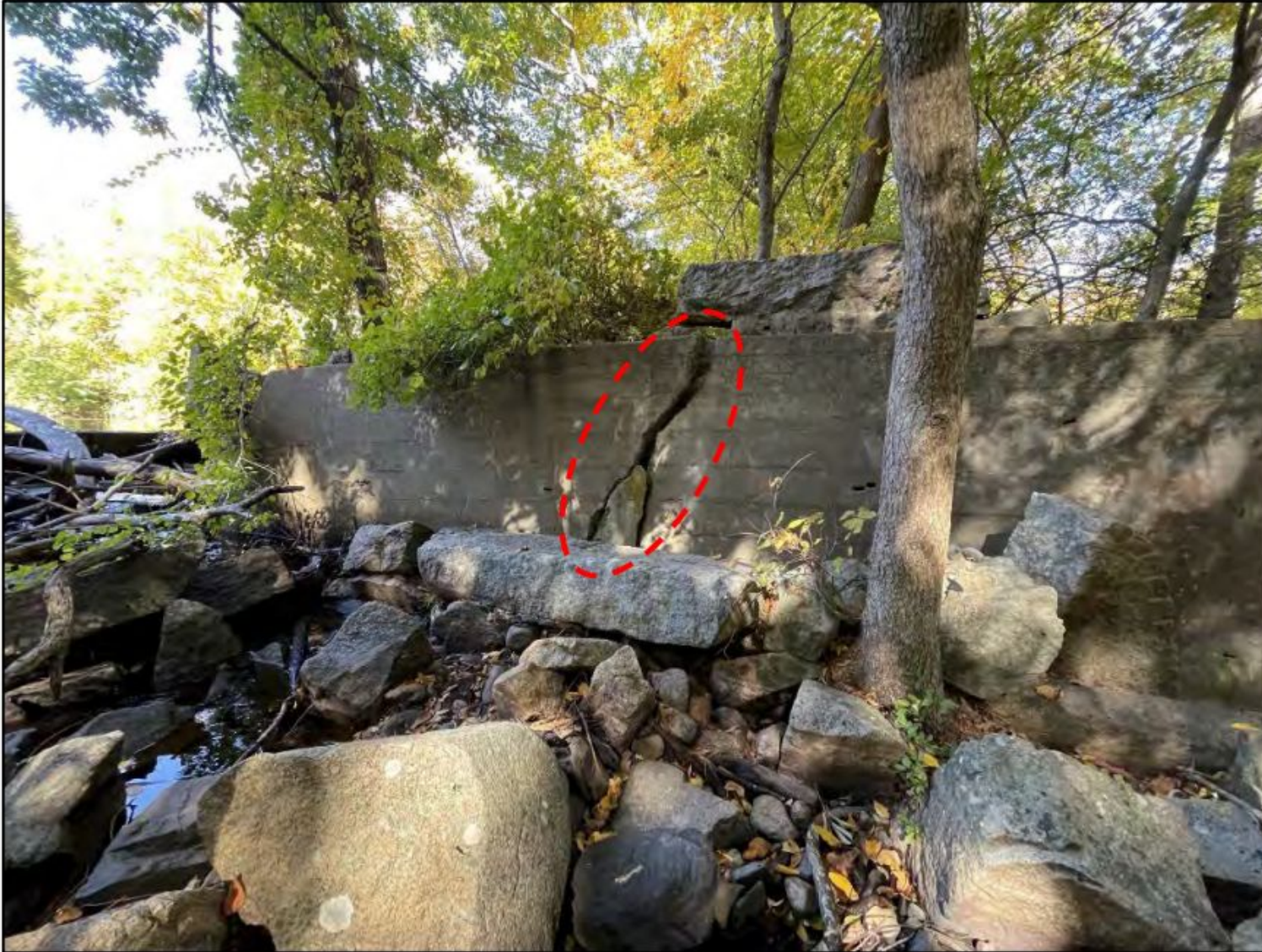
Photo No. 16.: Concrete wall left of the spillway. Note the 5-inch crack.
