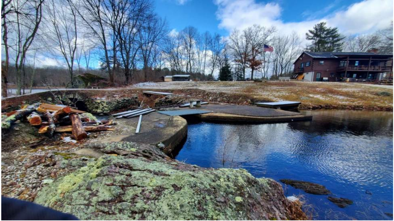
Photo 5: Unnamed dam at Mill Pond looking at the two auxiliary spillways from the right abutment of the primary spillway. The left auxiliary spillway is a stoplog-controlled channel, and the right auxiliary spillway is an earthen channel.
