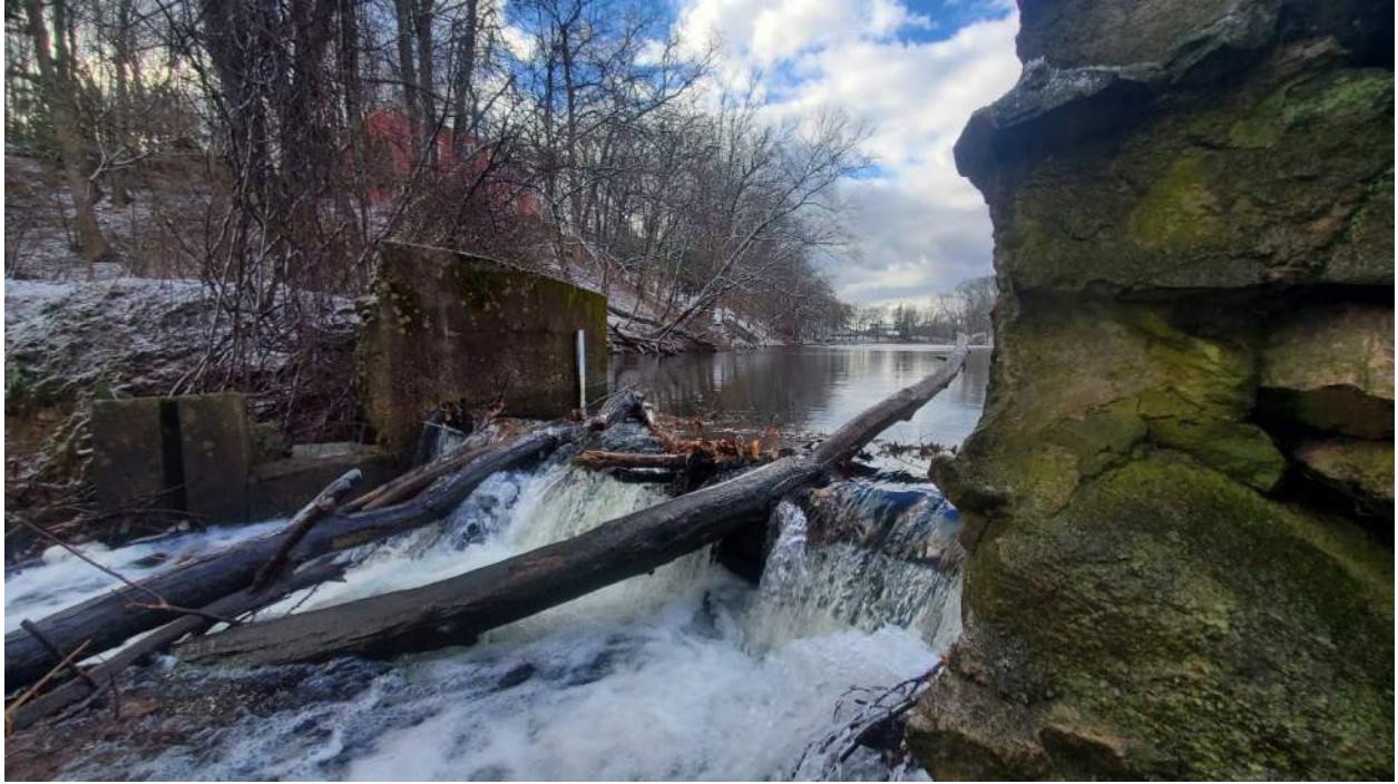
Photo 3: Eagle Lake Dam's (MA02263) primary spillway looking upstream. A staff gage is located on the right training wall.
