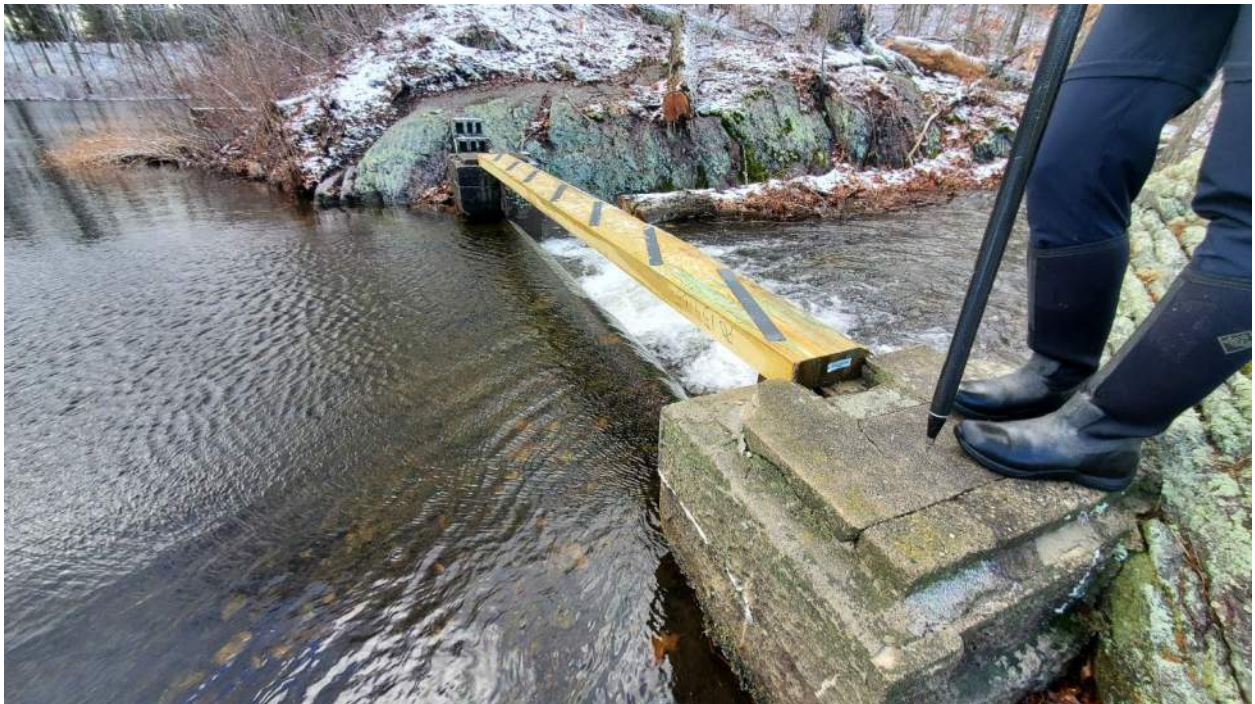
Photo 4: Unnamed dam at Mill Pond primary spillway. The primary spillway appeared to be a broad crested weir with a fixed angle iron.
