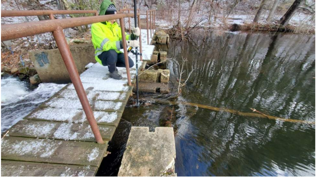
Photo 7: Bush Pond Dam (MA01158) looking at the spillways from the dam embankment. The spillways consisted of three stoplog-controlled channels.
