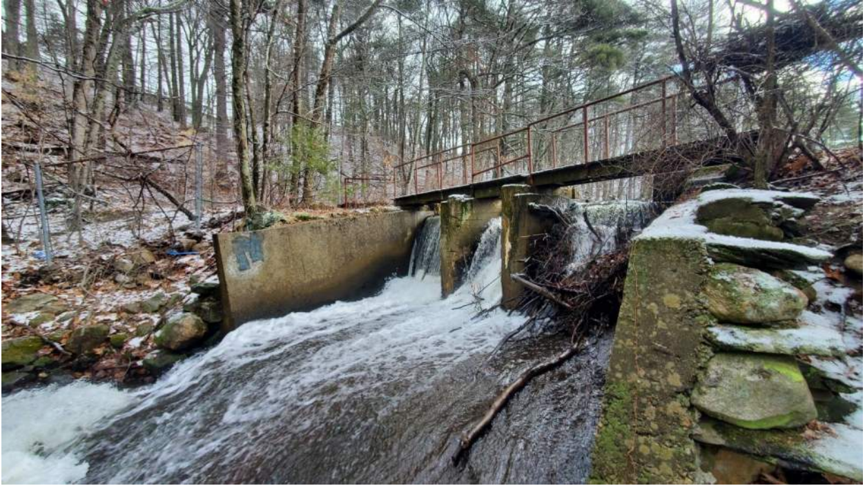
Photo 9: Bush Pond Dam (MA01158) looking upstream at the spillways from the toe of the dam.
