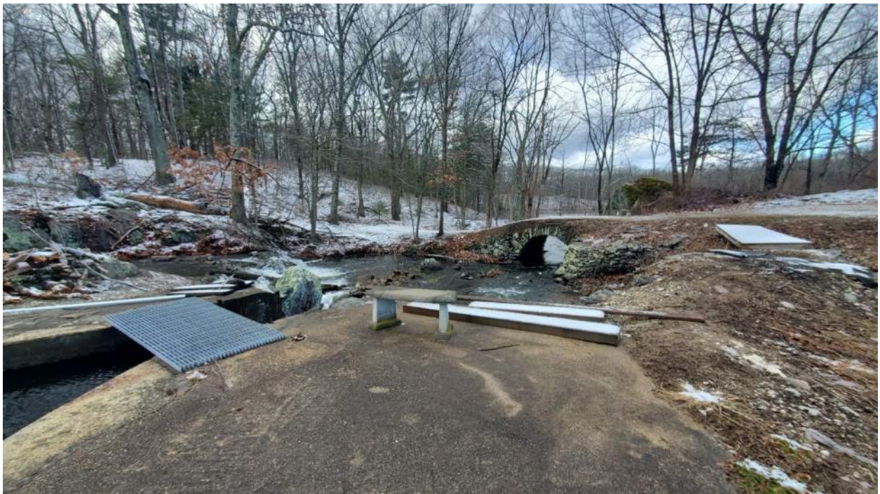
Photo 6: Unnamed dam at Mill Pond looking downstream at the stone culvert crossing downstream of the dam. The left auxiliary spillway is pictured above, with the right auxiliary spillway off-camera to the right.
